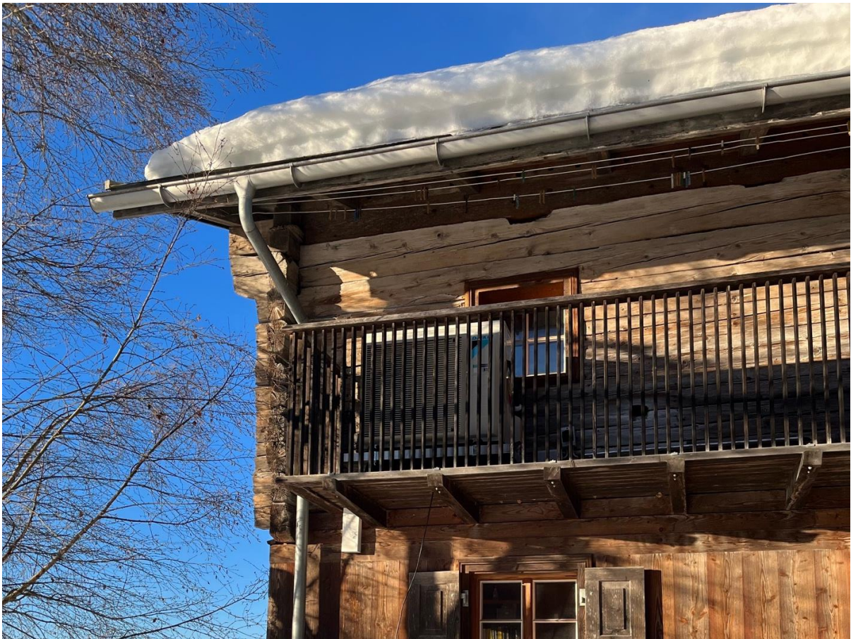
Figure 8: Outdoor unit on the left on the balcony (without visual impairment of the traditional building)
