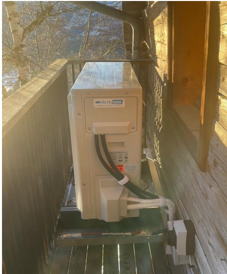
Figure 9: External unit of the AC
