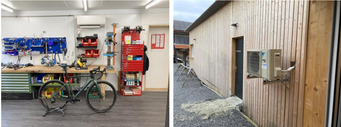
Figure 5: Bike repair shop: Indoor and outdoor units (Daikin). The air conditioning system is programmed the evening before so that the desired interior temperature prevails at the start of work.
