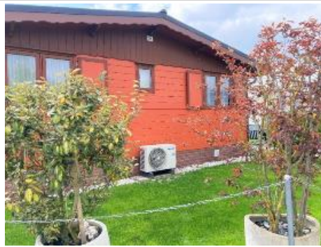
Mobile home, Fribourg, 4.0 kW
