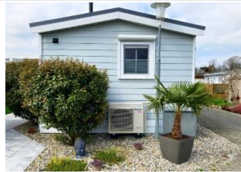
Mobile home, Fribourg, 5.2 kW
