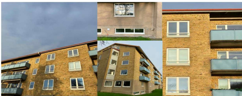
Figure 1 - newly installed energy efficient windows in Murödlan i Bö, a housing cooperative in Göteborg.
